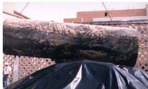
↑ 20,000 Gallon UST Being Removed from International Paper Facility in San Antonio, TX.
