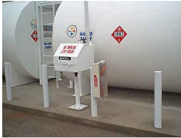
↑Aboveground Fuel System at Judson ISD Transportation Facility in Converse, TX.
