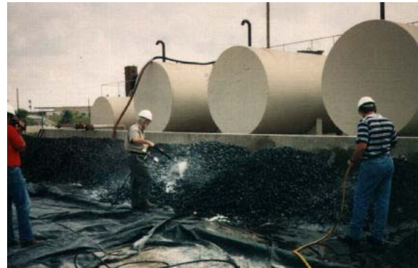
↑Diesel Spill Cleanup at Union Pacific Yard in South TX.
